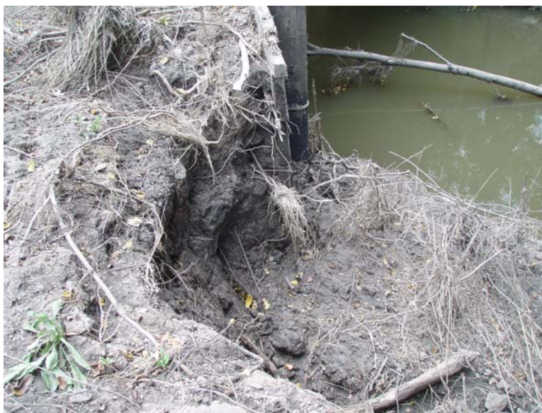
EROSION AT NORTHEAST CORNER
