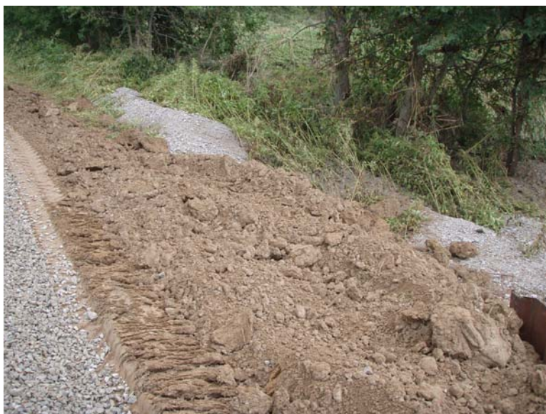
ROCK LOSS NORTHEAST CORNER
